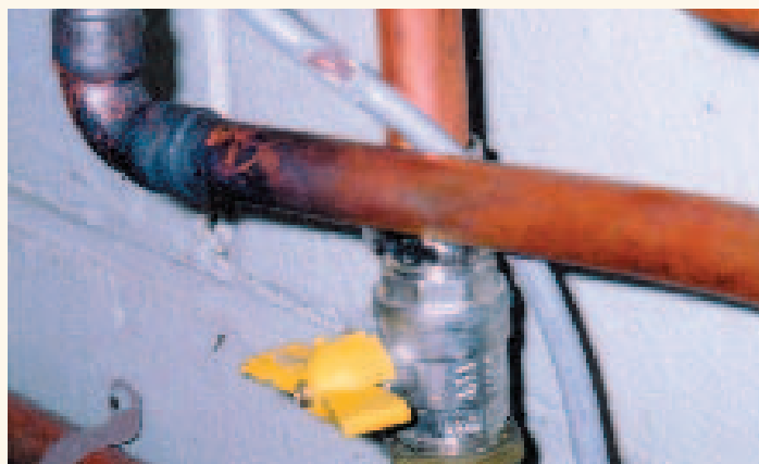
The power cord draped over the hot and cold water pipes.
