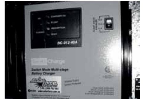
A battery charger not displaying evidence of approval
