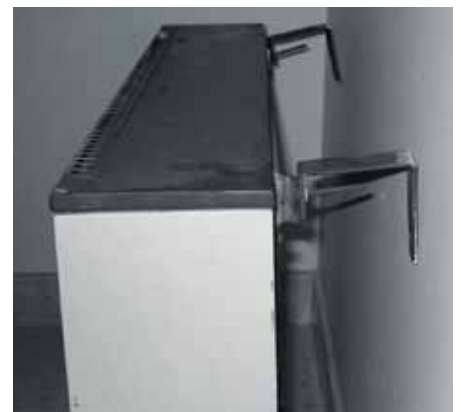
A flueless gas heater can look like any other when viewed from the front – but side on one can see there is no flue.
