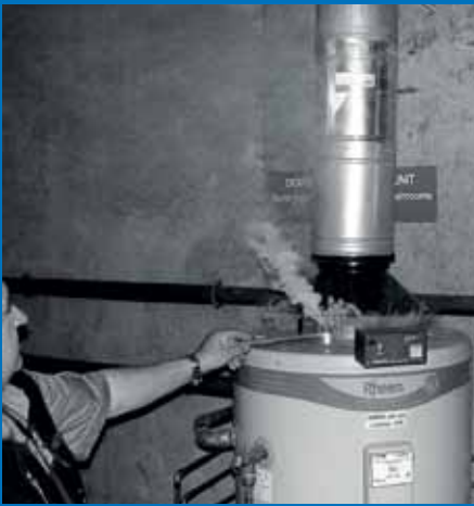
Gas Inspector Sam Zappulla conducts a test of a gas appliance in a plant room.
