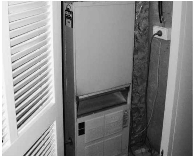
Gas unit, Lansell Road, Toorak.
